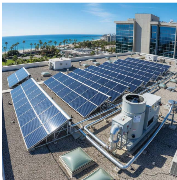
Hybrid hot water systems combining solar thermal and heat pump technologies drastically reduce energy consumption in hospitality operations.
