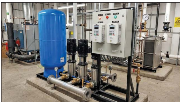
Hydropneumatic systems maintain constant water pressure in high-rise hotels while reducing the need for large rooftop storage tanks.
